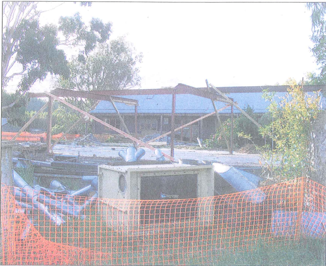
Knocked down: Hohepa's woodwork building has been demolished after sustaining damage in the Canterbury quake.
