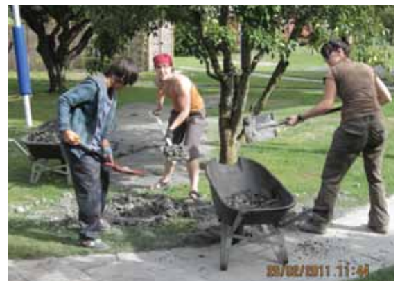
Volunteers came to help us shovel silt
