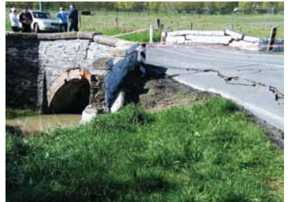
Farm access bridge damage
