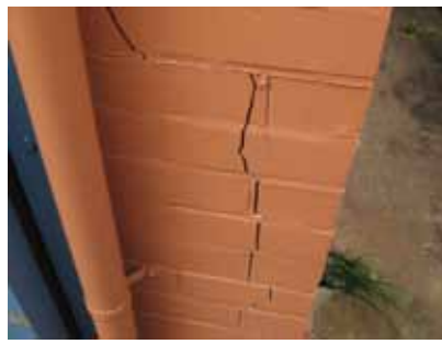
Damaged Sloss House showing cracks
