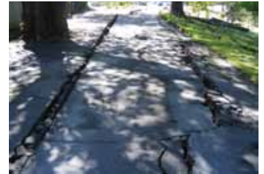
Damage to Barrington Street driveway following February 22 earthquake.
