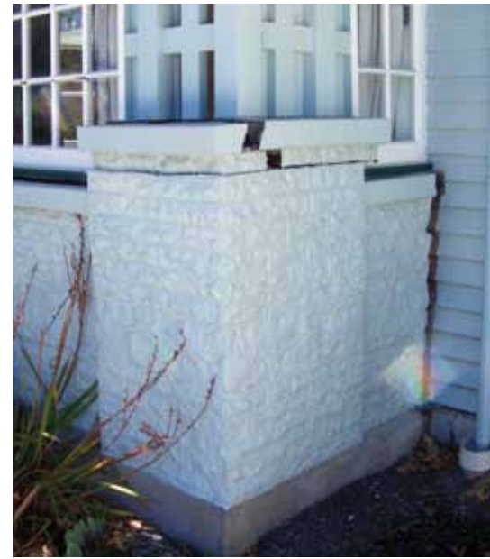
Damaged Jade House
