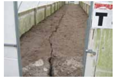
Lateral fracture running the length of the tunnel house
