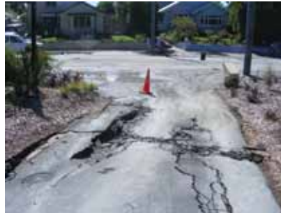
Silt and driveway cracking in Barrington Street from February 22 earthquake
