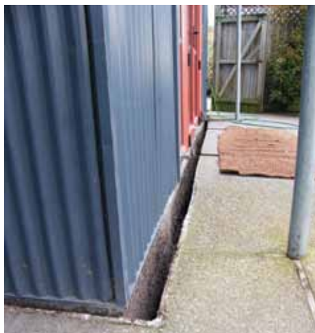
Farm Day Base showing movement on foundations
