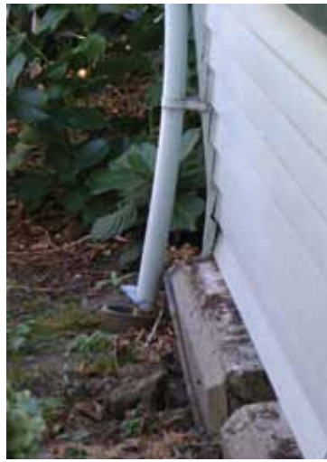
Jade House earthquake damage
